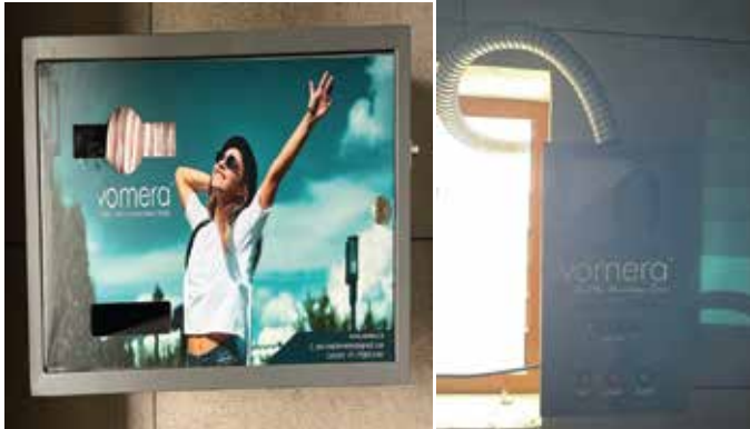
Sanitary Napkin Incinerator and Vending machine was installed at the K-DISC Innovation Tower in connection with the Womens' Day celebrations followed by a cake cutting of Women Employees at our Headquarters.
