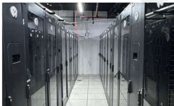
Fig. 11.3 KGDC Facility at Digital University, Kerala
