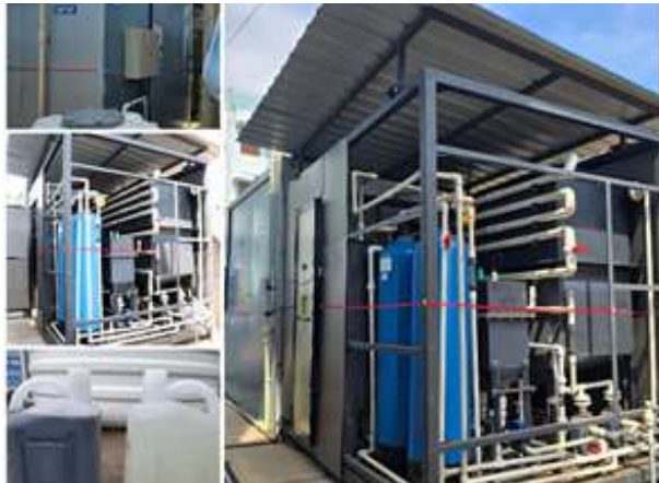
Fig. 5.2 35KLD decentralized STPs using biofilter & electrochemical technologies installed for 110 fisher families at Vizhinjam
