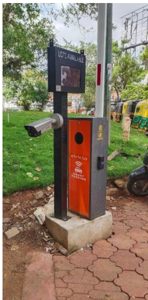
Figure 44 ANPR Camera and Boom barrier installed at Gandhi Park, Thiruvananthapuram
