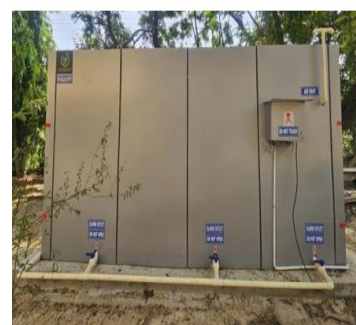
Figure 28 OLOI - Decentralized Sewage Treatment Plant 2
