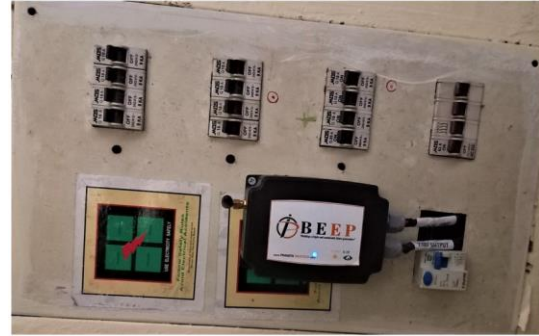
Figure 87 BEEP device installed next to a distribution board at a premise
